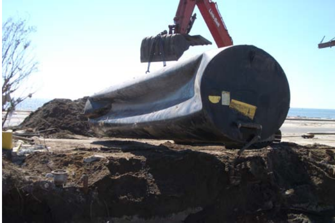
Collapsed gasoline tank. Hurricane Katrina – 2005, Biloxi, MS
