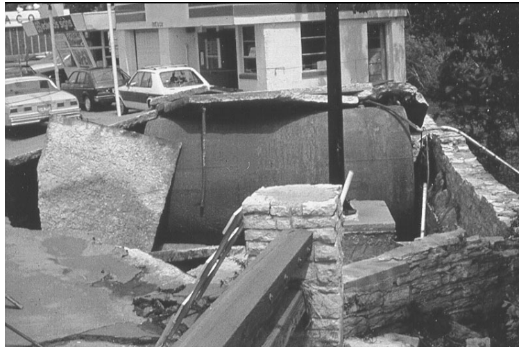
UST lifted by buoyant force
